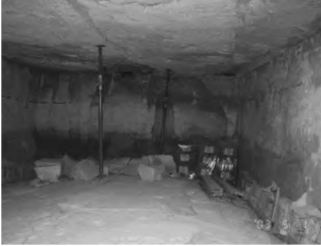
Figure 50. The uplifting of soft-limestone layer due to swelling of Esna shale beneath in the tomb of Ramses II.
