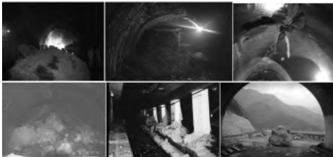
Figure 41. Views of damage to tunnels in recent earthquakes.
