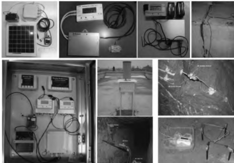
Figure 36. Views of multi-parameter system and its in-situ set-ups.
