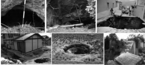
Figure 42. Views of sinkholes above karstic caves and abandoned lignite lines in recent earthquakes.
