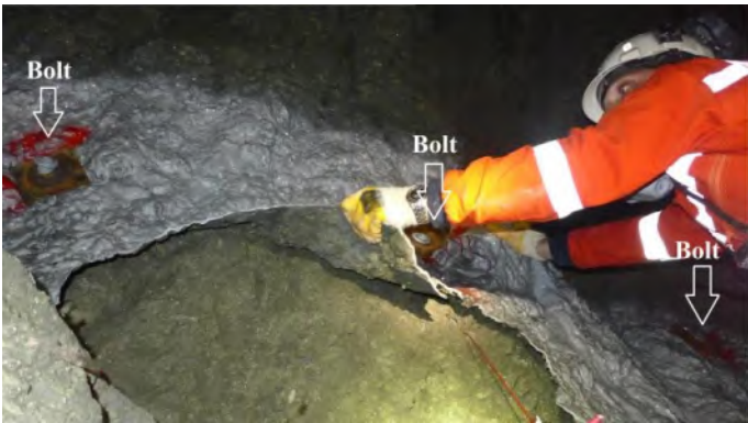
Figure 11. Failure of the TSL with 3 mm thickness (No failure at bolt plate parts)
