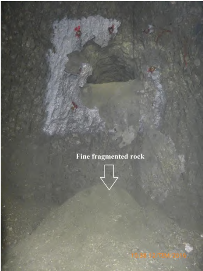
Figure 7. Rock accumulated in front of the face
